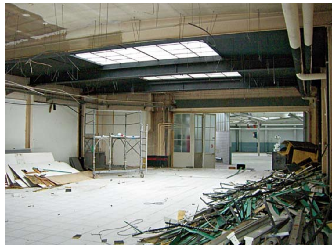
THE VON BARTHA GARAGE DURING THE RENOVATION, JULY 2007 PHOTO BY LUKAS VOELLMY
